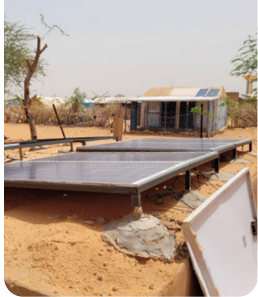
Solar panels in need of maintenance
