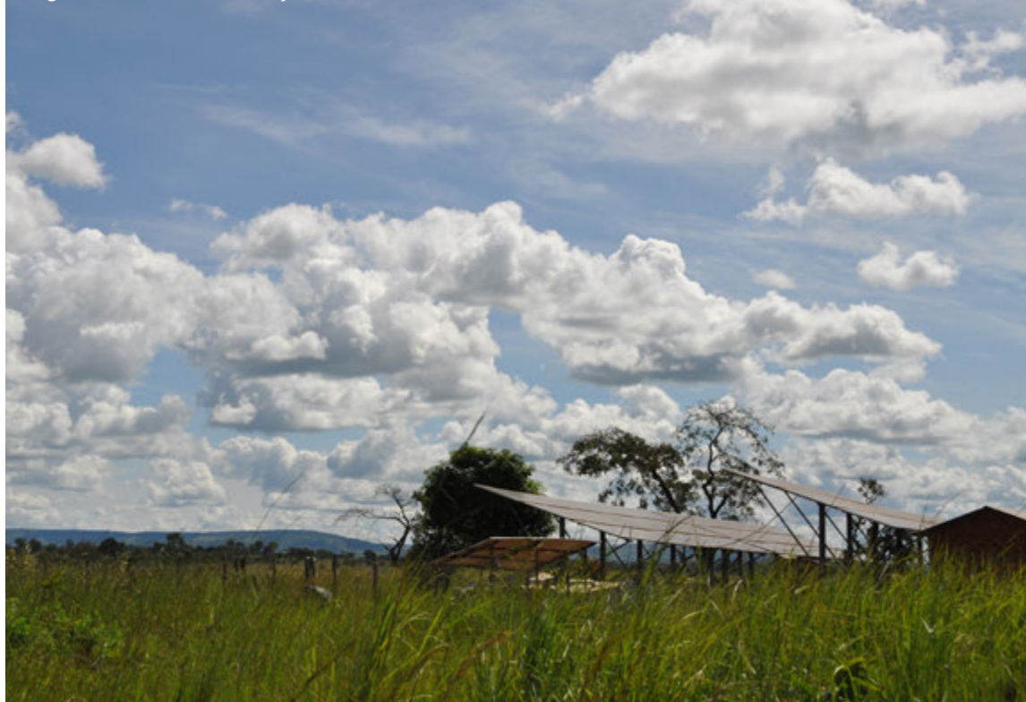
A ground-mounted solar system
