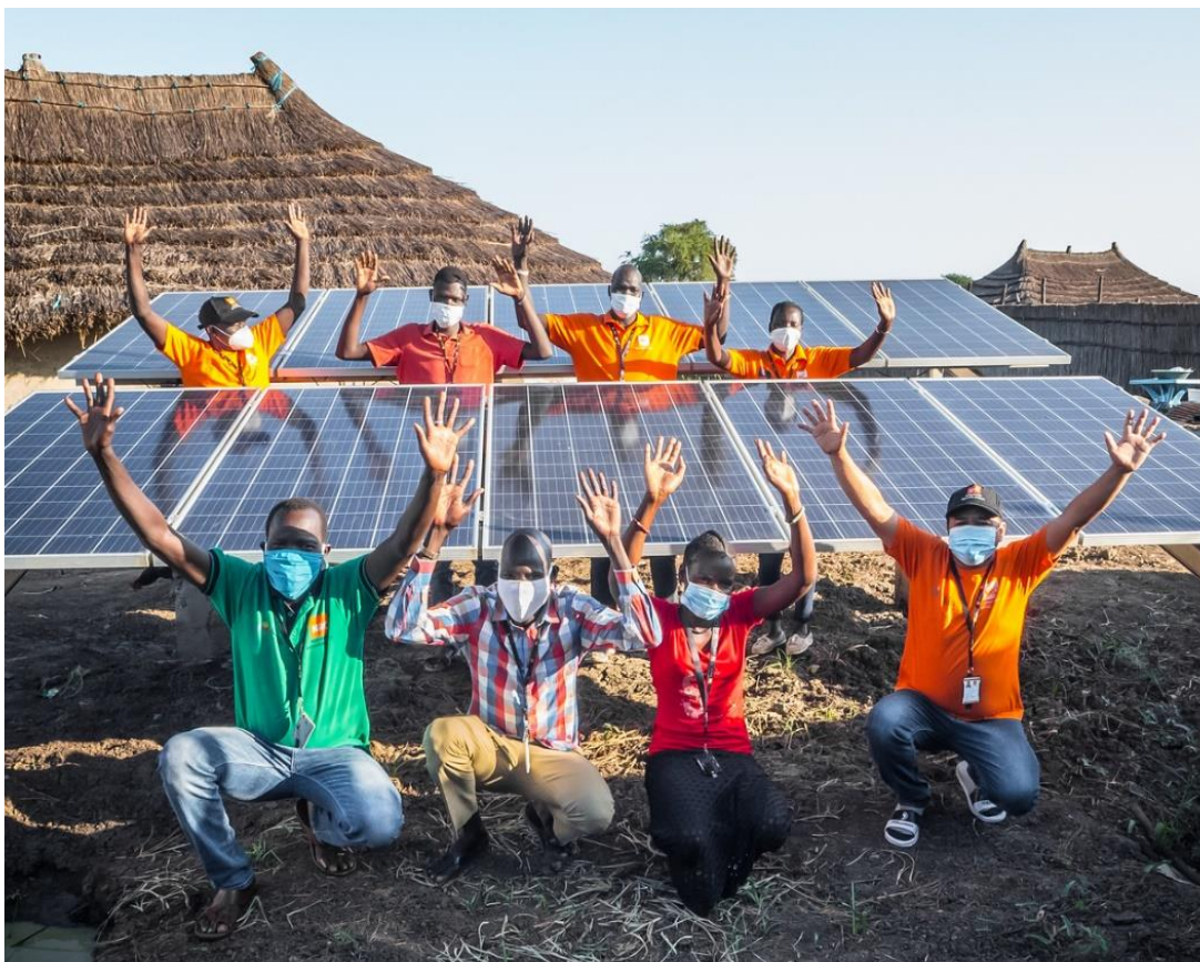
In 2020, solar panels were installed at the NRC office in Mankien, South Sudan. The team now have their own power supply and enjoy renewable energy 24/7. Photo: Iban Colón/NORCAP
