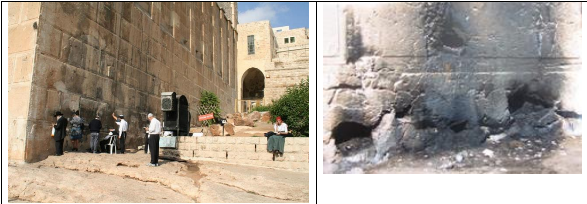
Figure 7: : Historic stones at the eastern façade of the Mosque are damaged due to the misuse of the Israeli settlers lighting candles while praying
