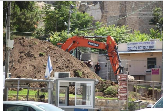
Excavations works by the Israeli authorities in the front yard of the Ibrahimi Mosque to construct the elevator
