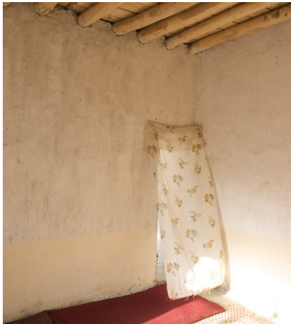
An alternation put in place by several beneficiaries was a door at the back of the house, linking it to a cleaning / toilet area. However the position of such door (by the corner) is a potential threat to the stability of the house.
