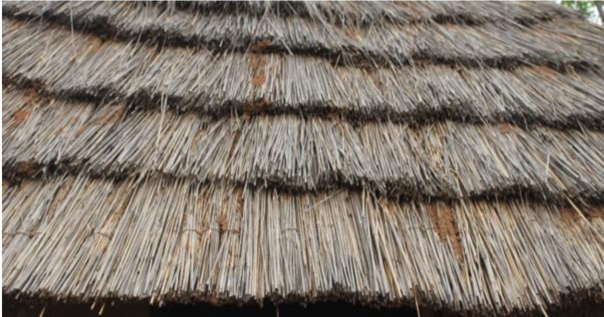
Picture 3 - A grass thatch roof under attack by termites in Kule camp, Gambella, barely a year after construction. Picture by Timothy Mutunga, May 2015
