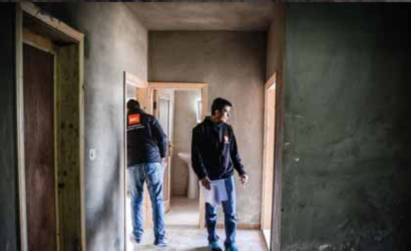
NRC's engineers visit a property registered with our urban shelter programme in Irbid governorate, Jordan, to consider when it is ready to be moved into. Photo: NRC Jordan/Dara Masri
