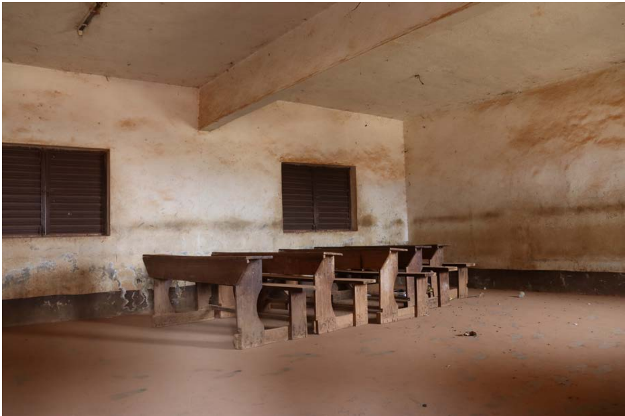
Abandoned school in the North-West region, Cameroon. (Photo: Bibiane Mouangue/UN OCHA)
